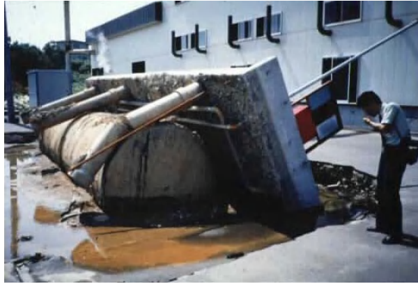
Empty tank floated up in 1993 Hokkaido Nansei-oki Earthquake
